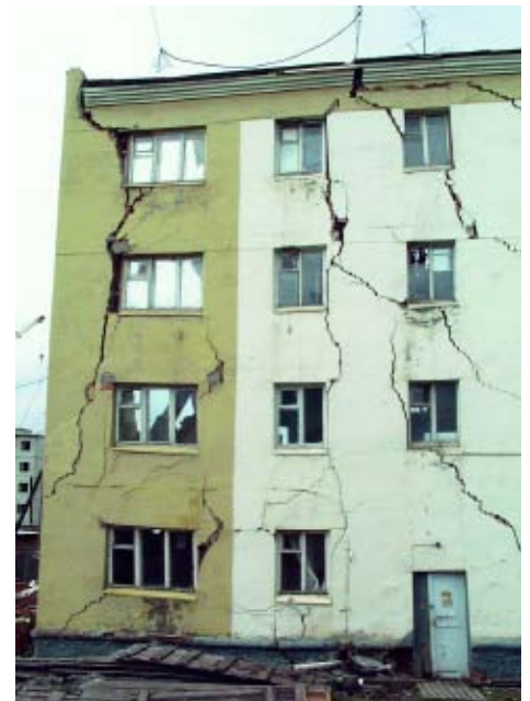
Building damaged due to permafrost thawing in Chersky (low Kolima River), Russia.
