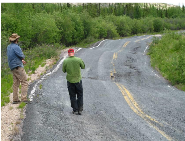
Thawing permafrost damaged this section of Highway 4, east of Yellowknife in Canada’s Northwest Territories. Photo credit: Natural Resources Canada.
